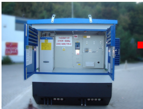
Transformer station HV/LV
